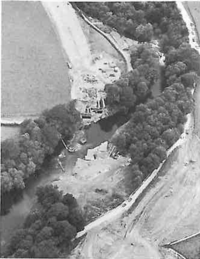
Above:— An aerial view of the site of the Kent Bridge and road construction proceeding North towards Brettargh Holt Interchange. The piers and abutments rise from the river and the N.C.K.605 assists with the installation of temporary foundations in midstream to carry supports to the Bailey Bridge which will be used in the casting of the 195ft. main span.
