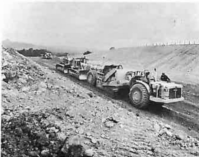
Below:— Bulk earthworks are well advanced towards a substantial completion by the end of October. Here a T.S.24 Motor Scraper is being tandem-pushed in excavating one of a number of deep cuttings with a high boulder content.
